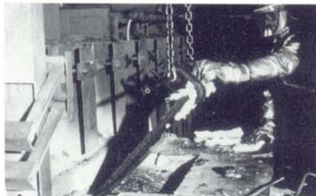
Figure 1: (a) A vertical gate filter (VGF) being installed into a reverberatory furnace dipwell.
