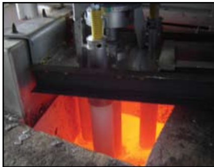
T-35SD circulation pump in side well furnace
