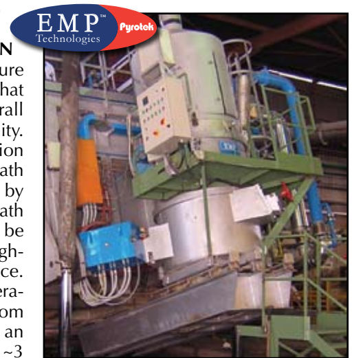
EMP pump and charge well on tilting furnace
